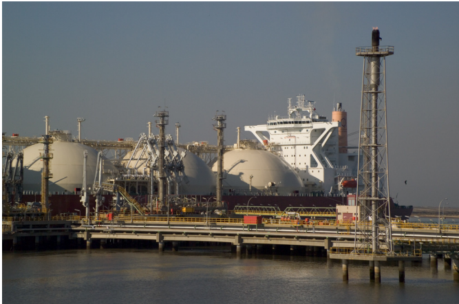
Figure 1: Unloading arms at the jetty in an LNG Receiving Terminal connecting the ship's tanks and the ground's tanks during a Custody Transfer process
